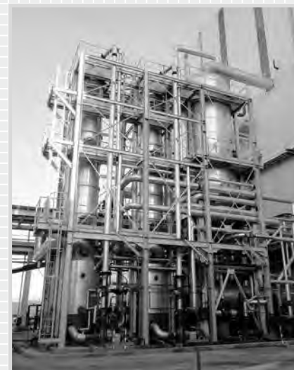
Design and installation of evaporation station for La Belle Sugar Refinery in Algeria
