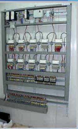
Mounting of switchboard for boiling house automatic control system
