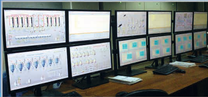
Main operator's room at Gaysyn Sugar Plant (Ukraine)
