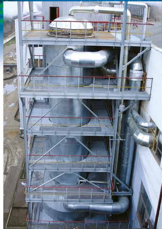
TVP 12-4870 Evaporator (Skidel Sugar Factory)
