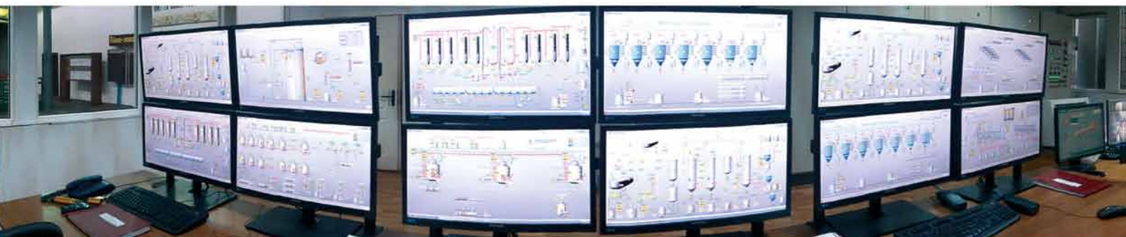
Main Operator's Room at Sugar Plant (Gaisyn Sugar Plant)
