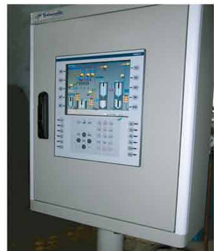
Purification Station Control Operator Panel
