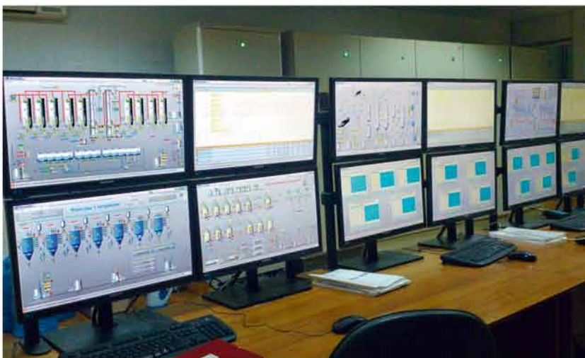
Main Operator's Room at Sugar Plant
