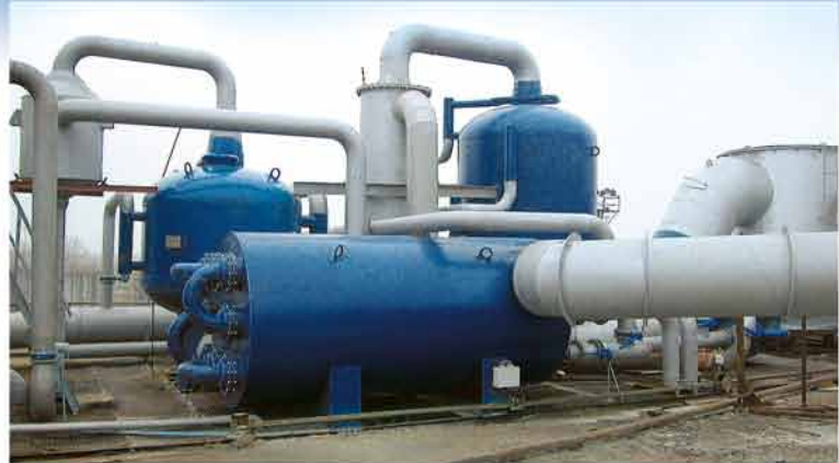
Vacuum Condensing Unit at Volodymyr-Volynsky Sugar Plant
