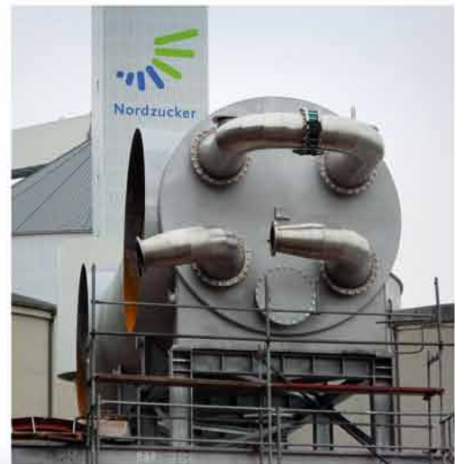
Raw Juice Heater Mounted at the Uelzen Nordzucker Refinery
