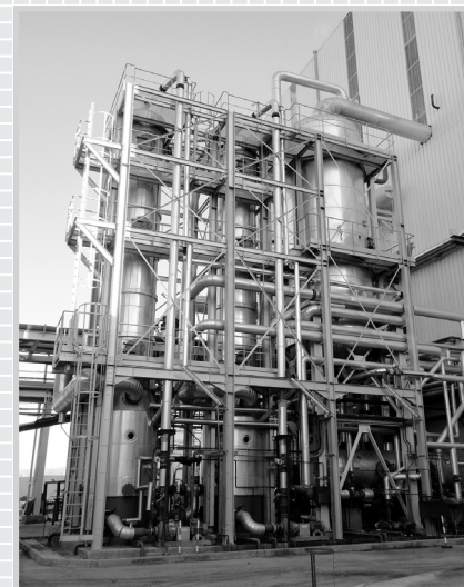
Design and installation of evaporation station for La Belle Sugar Refinery in Algeria
